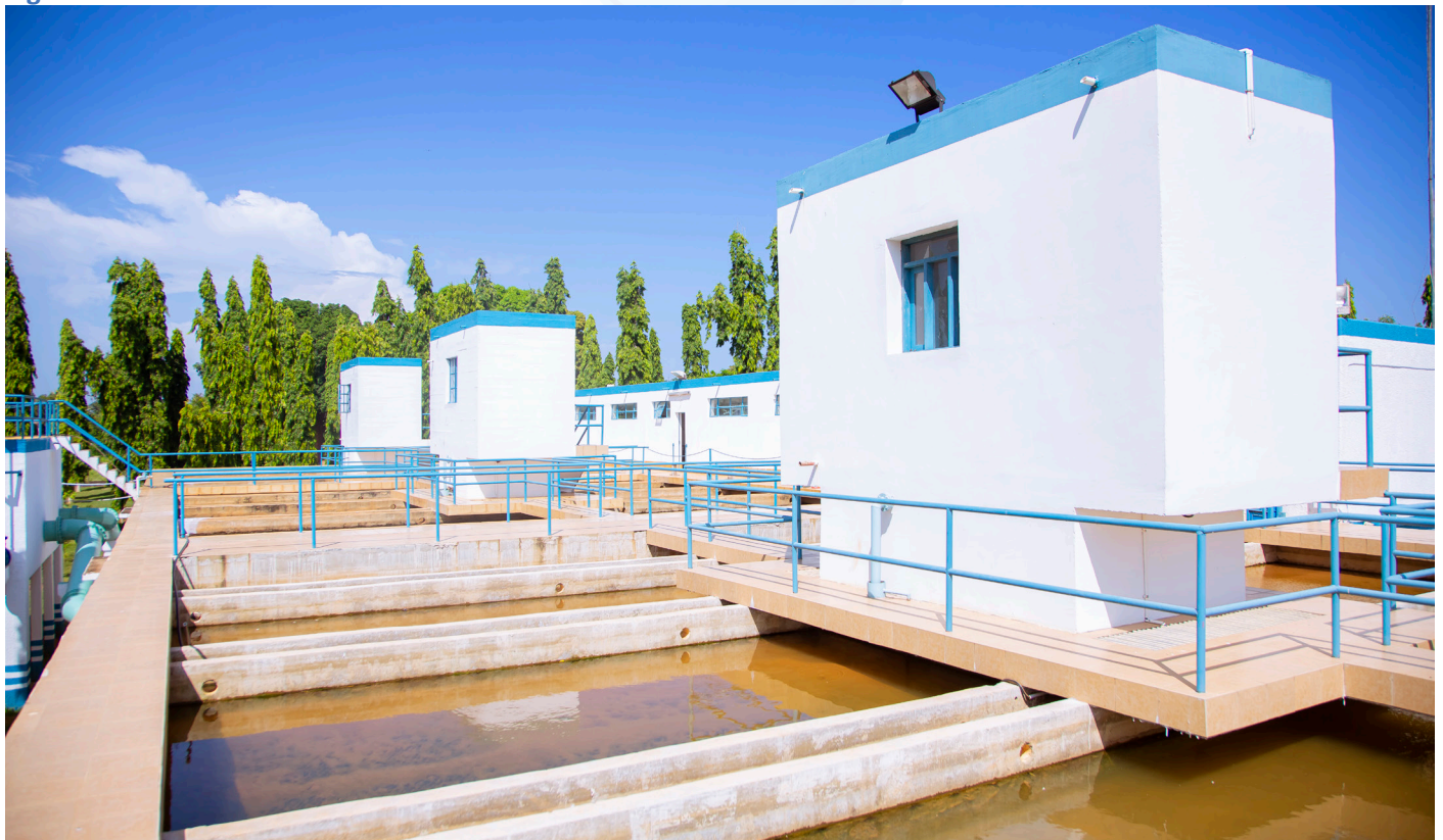
Figure 14: Flocculation Tanks at Mowe Water Treatment Plant
